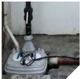
-1. kat zeminine kurulan SANICUBIC 2 VX
