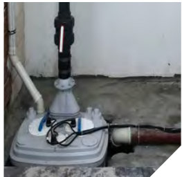
-1. kat zeminine kurulan SANICUBIC 2 VX
